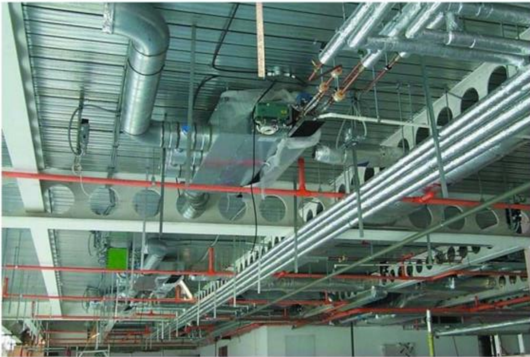
Coordination between ductwork and structural element
